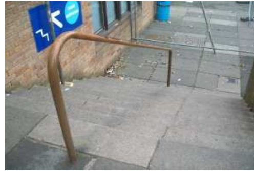
External Stairs (Limited Handrail Provisions)
