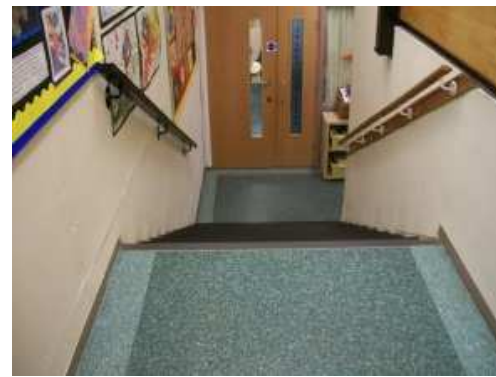
Poor Handrail to Internal stair Leading to Nursery
