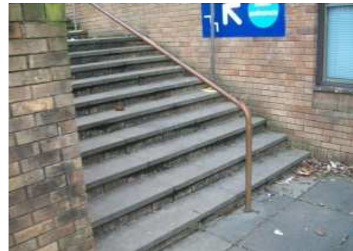
No Markings to External Stairs
